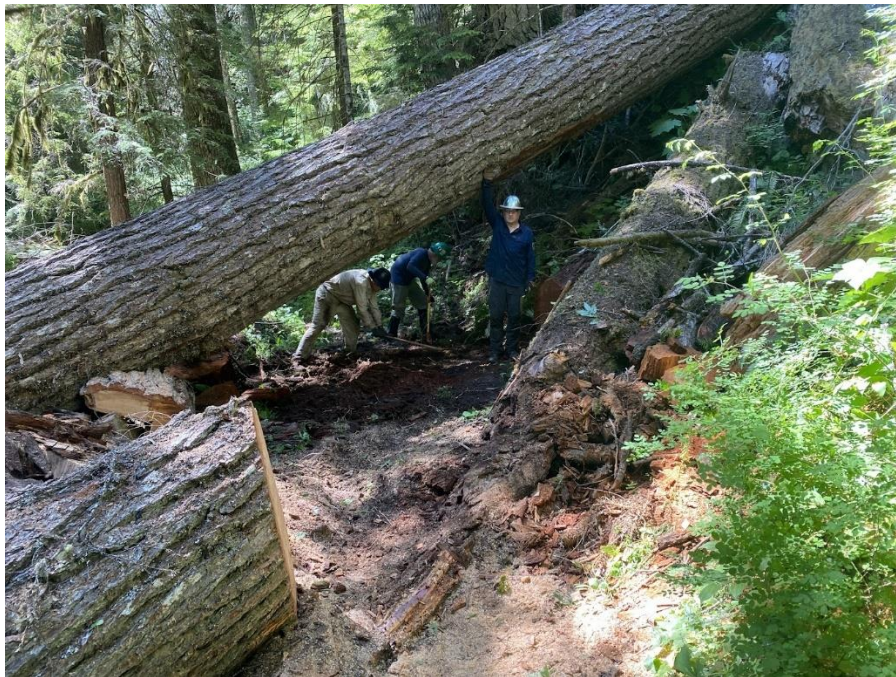
JUMBLED LOG MESS: AFTER. WE OPTED TO LEAVE THE OVERHEAD LOG FOR SEVERAL REASONS, NOT THE LEAST OF WHICH IS THAT THE COSTS OUTWEIGHED THE BENEFITS. THERE IS A 7-FOOT CLEARANCE SO, AT MOST, A RIDER WOULD HAVE TO LAY DOWN OR DISMOUNT. BUT EVEN A TOOL-LOADED MULE COULD PASS UNDER THIS. OUR TREAD TEAM CAME ALONG JUST IN TIME TO MOVE THE TRAIL FURTHER UP TO PASS UNDER THE HIGHEST POINT.
