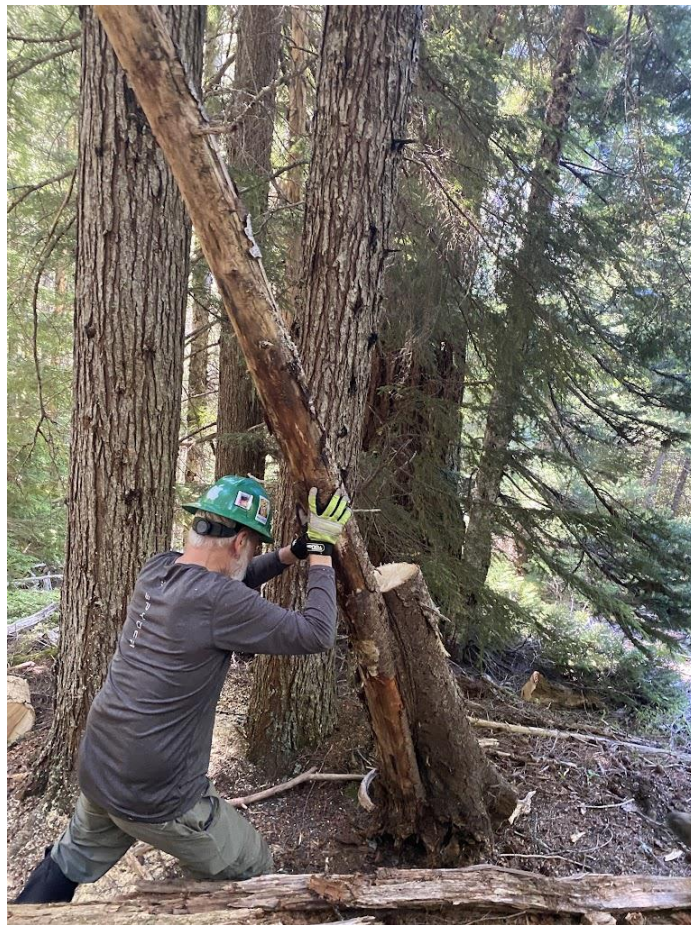
BRIAN AND DAVID DID NOT HAVE PRESSING TREAD WORK UP HERE, SO THEY CARRIED TOOLS AND GAS, AND MOVED ALL THE CUT PIECES OFF THE TRAIL.
