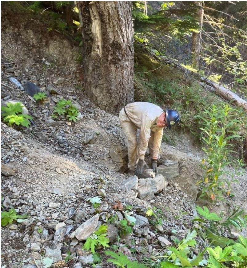
YET ANOTHER ROCK FORTIFICATION PROJECT. THIS WAS AT THE TOP OF A GULLY WHERE YOU DO NOT WANT TO SLIP AND FALL.
