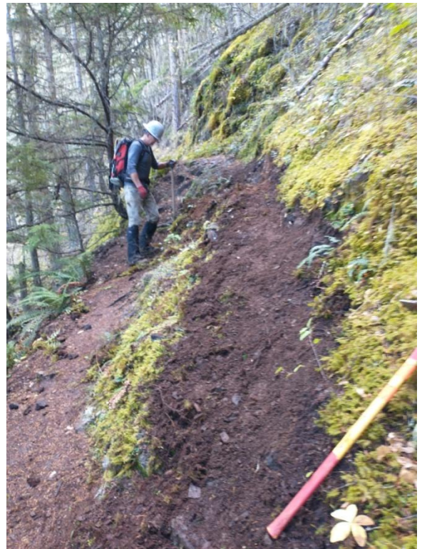
rough bypass of lower section that's moved down-slope and ends in 3ft step
