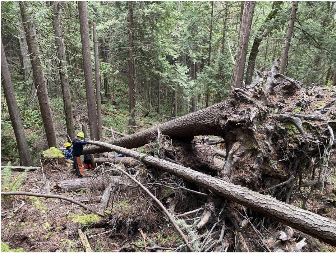
Randy and Nate looking over the project, discussing all the aspects of the situation in terms of OHBEC (that's Objective, Hazards, BINDS (usually "Leans" but that's for felling, which we were not doing), Escape Route and Cut Plan. Note the snag that is to the right of Randy's yellow hard hat. The students needed to recognize that as a hazard and ask Martin (who is certified for felling) to cut it down. That was done.
